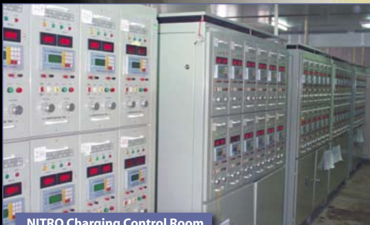
NITRO Charging Control Room
